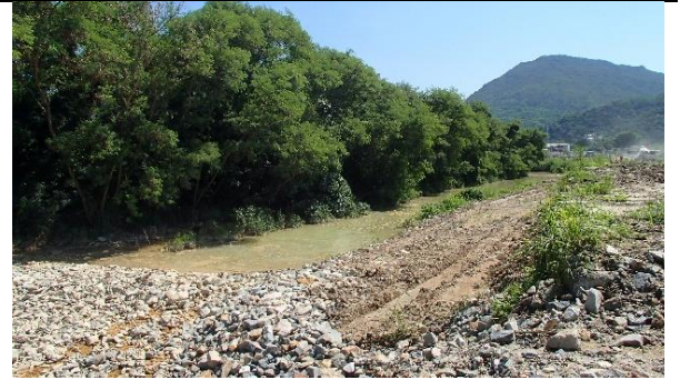
Drainage channel in TKO Area 137
