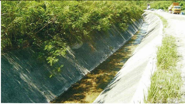
Drainage channel in TKO Area 137
